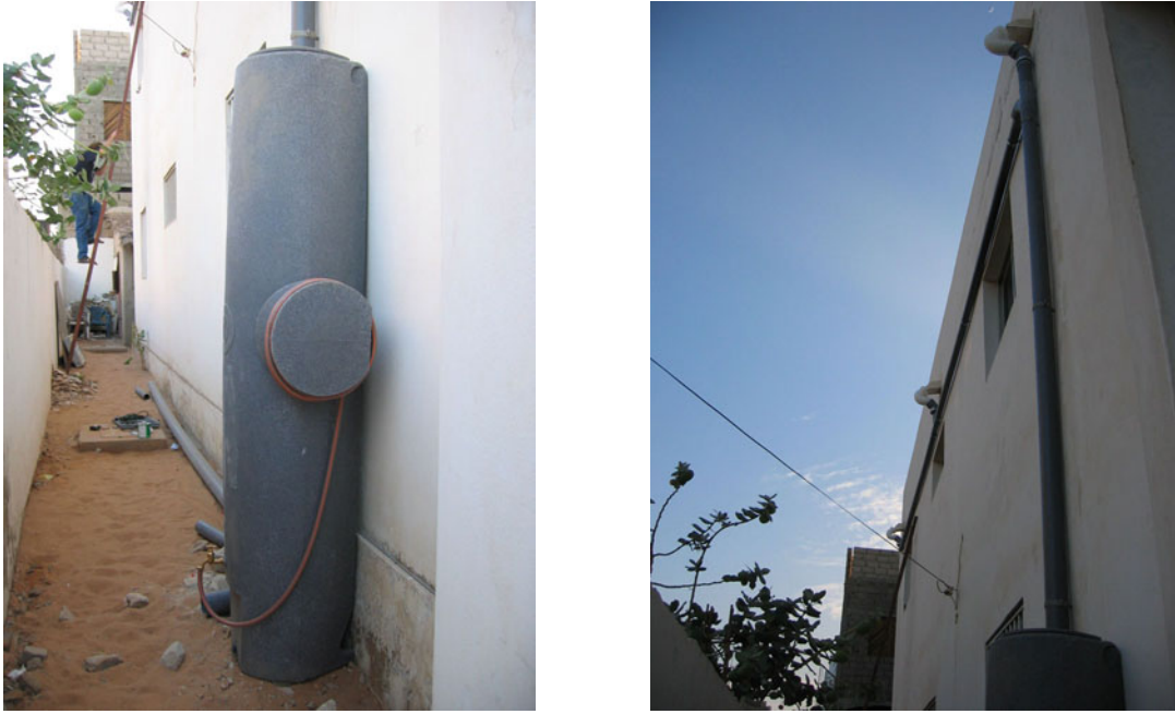
Figure 20: Rainwater Collection Tank (left) and Piping System (right)
